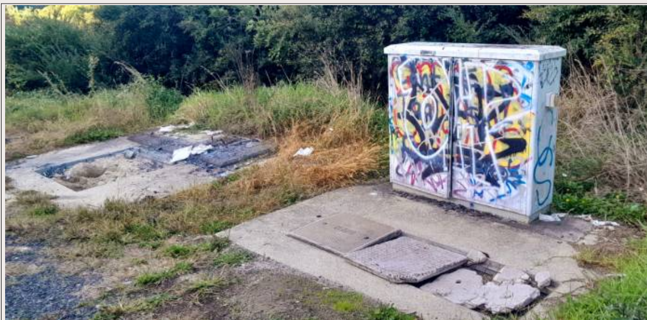
Above: Total destruction of our phone/internet cabinets down at Hangapi Rd (JS)
